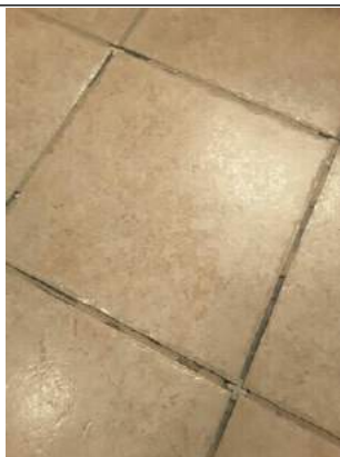
Floor was in need of some grout repairs.
