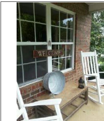
Missing window screen. Front porch.
