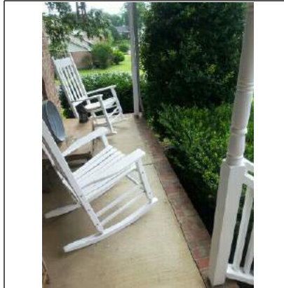
Recommend handrails on a porch over 36 inches off the ground.
