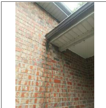
Same place where there is no kick out flashing. Water runs down the brick wall instead of in the gutter.
