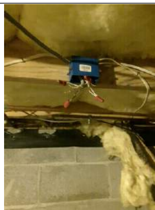
Open junction box in crawlspace. Recommend licensed electrician repair.
