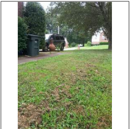
Negative grade at southwest side of house by driveway. Maybe 2%. With a heavy rainfall, it may be possible for water to enter the garage. By adding downpipe extensions, it will significantly improve water dispersion away from the house.
