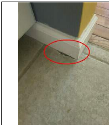
Gap between floor and wall.
