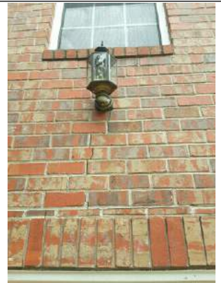
Step cracks above garage door. Recommend structural engineer evaluate.
