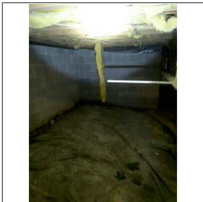
Loose and falling insulation batts. Recommend adding supports.
