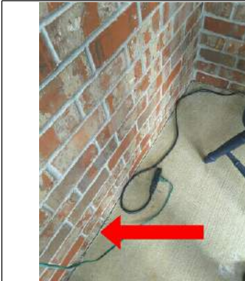
Recommend sealing gap between concrete and brick wall.
