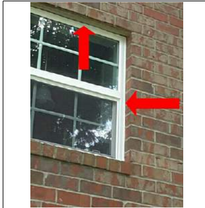
Caulking needed at windows.
