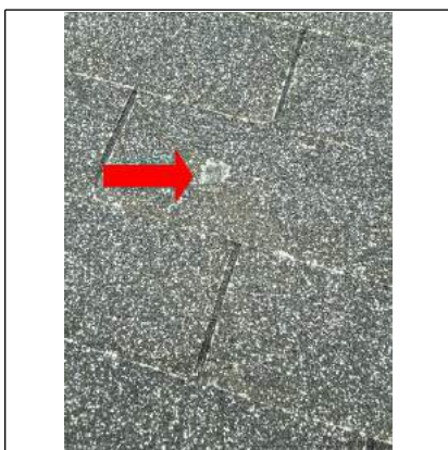
Notice the fiberglass showing through the shingle. There are also some hail damage spots.
