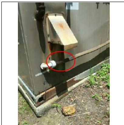
The flexible conduit directly under the exhaust flu of the HVAC unit needs repair...open.
