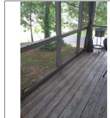
Missing balusters. Safety Hazard.
