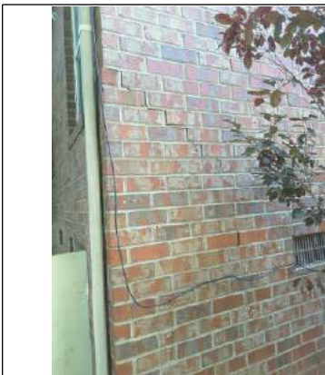
Northwest corner step cracks. The block foundation wall in the crawlspace behind this brick veneer also has a step crack. Have structural engineer evaluate.
