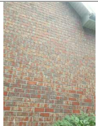
West wall step cracks. There is no bowing on this wall. I assume the cracks are from settlement due to water not being diverted away from the house properly for years.
