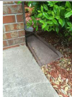
Recommend adding downpipe extensions to divert water away from foundation. 5-6 feet.
