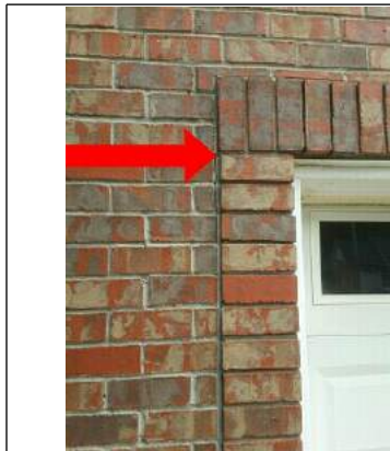
Small crack at mortar joint. Recommended repair.
