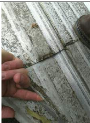
Open valley. Recommend licensed roofer evaluate/repair. I could easily slip my finger under the metal roofing next to the valley. The caulk here has failed.
