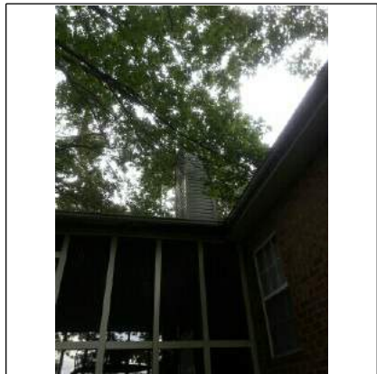
Recommend trimming trees that are in contact with the house or roof.
