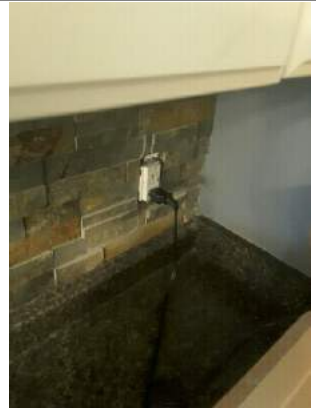
Cover plate missing. When GFCI trips, it is a combination of resets to properly reset each one on the wall with the sink.
