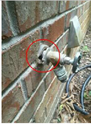
Loose hose bib on the west side of the house. Recommend sealing gaps.
