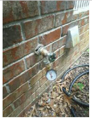
Hose bib is loose and the handle is leaking. You have 90 psi water pressure. This is on the west side.
