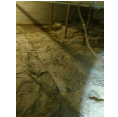
Some areas of the floor had no vapor barrier present.
