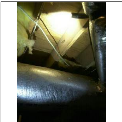
Missing floor insulation in crawlspace.
