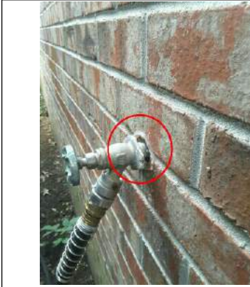
Loose hose bib on the east side, it also needs sealant in/around the hole.
