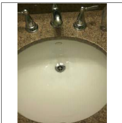
Missing drain plug in sink.
