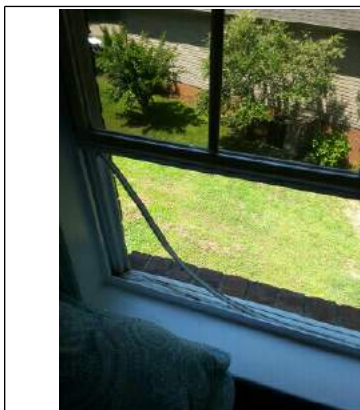
Loose weatherstripping on bedroom window.
