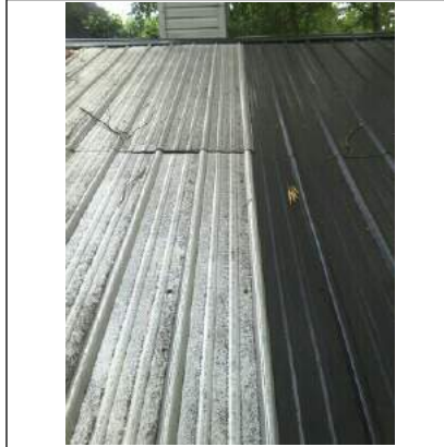
Metal roofing. This is over the deck. Some caulking has been applied to possible past trouble areas mostly around chimney.
