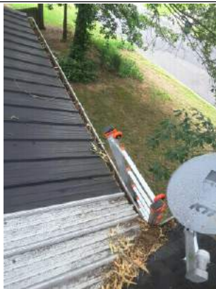
Gutter and Valley need to be cleaned.
