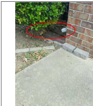
Downpipe extension needed next to garage. This will help to keep heavy rains from entering the garage.
