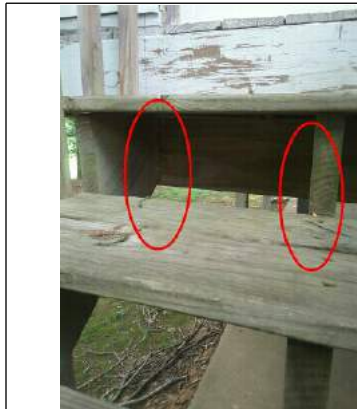
Steps not attached properly to deck. Recommend adding additional hangers.
