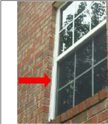
Caulking needed at windows.
