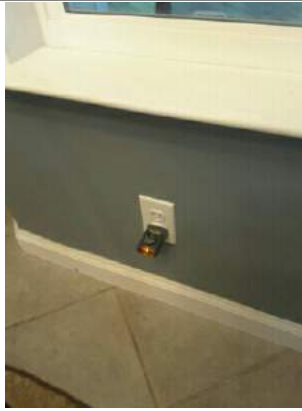
Open ground at breakfast area. Recommend licensed electrician repair.
