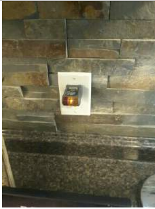
Faulty GFCI with an open ground. Safety Hazard.
