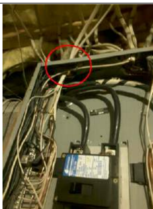
Missing protective grommet where Romex goes through electric panel. Recommend licensed electrician repair.
