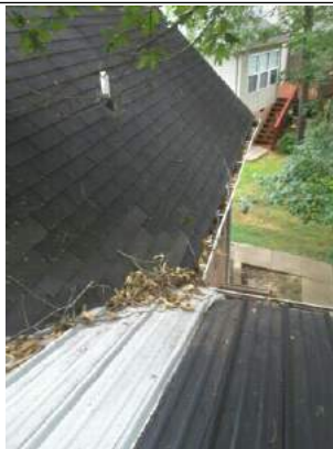
Valley and gutter on rear of house need to be cleaned.
