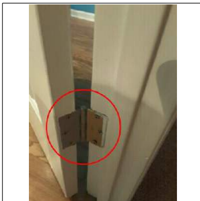
Loose hinge on bedroom door.
