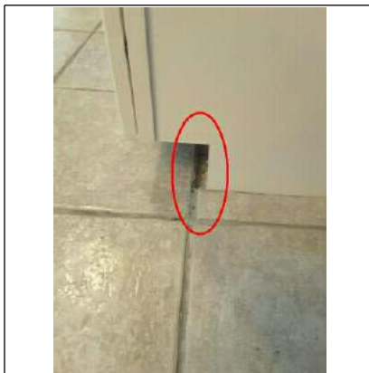
Gap between floor and cabinet base.
